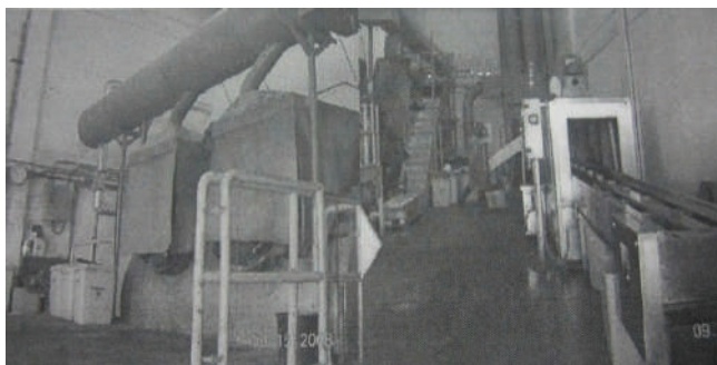
Figure 12. Treatment Facility (Company C).
