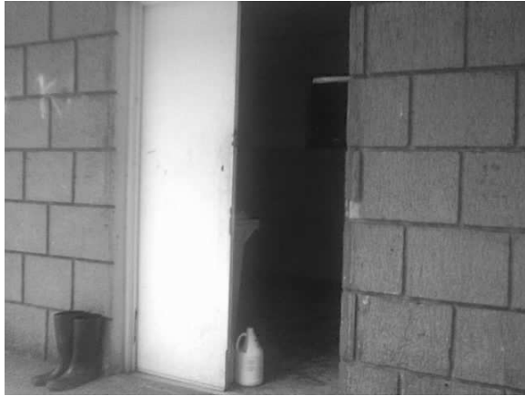
Figure 7. On-Site storage facility, Hospital B
